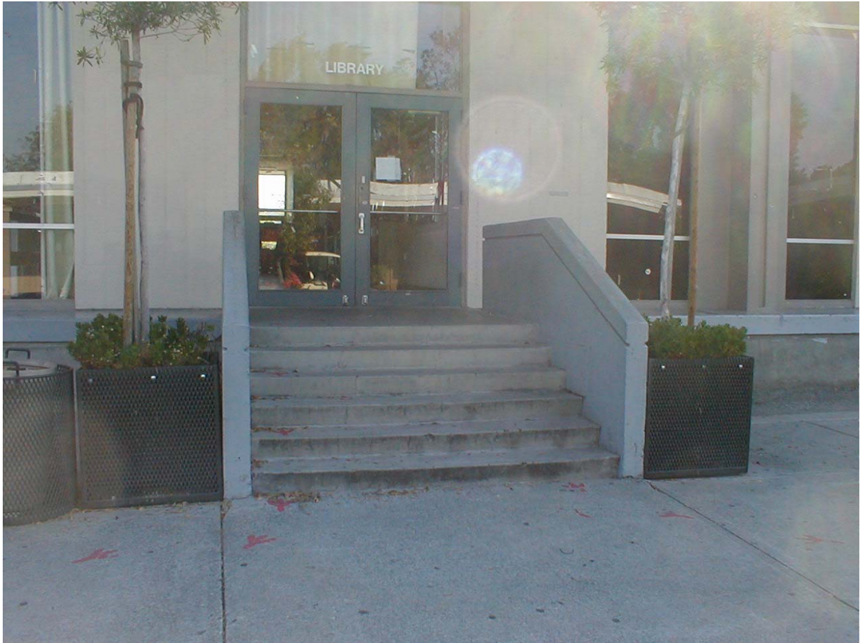
Nonconforming stair at library of Mt. Pleasant High School.
