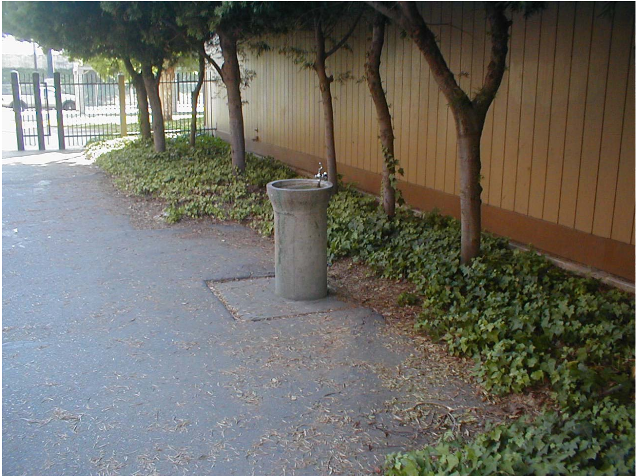
Nonconforming drinking fountain at Independence High School.
