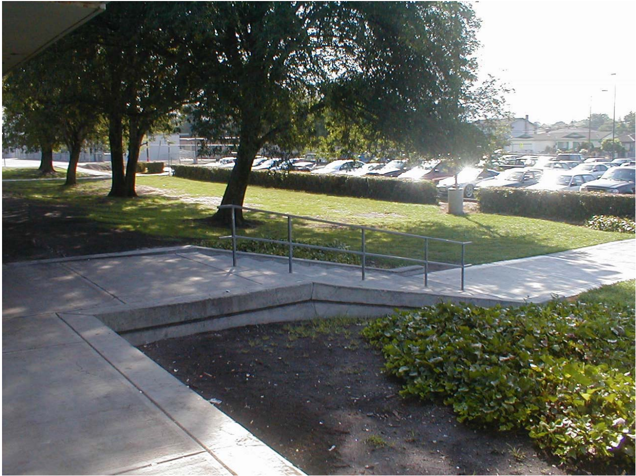
Nonconforming stair with no wheelchair access at main entry of Mt. Pleasant High School.
