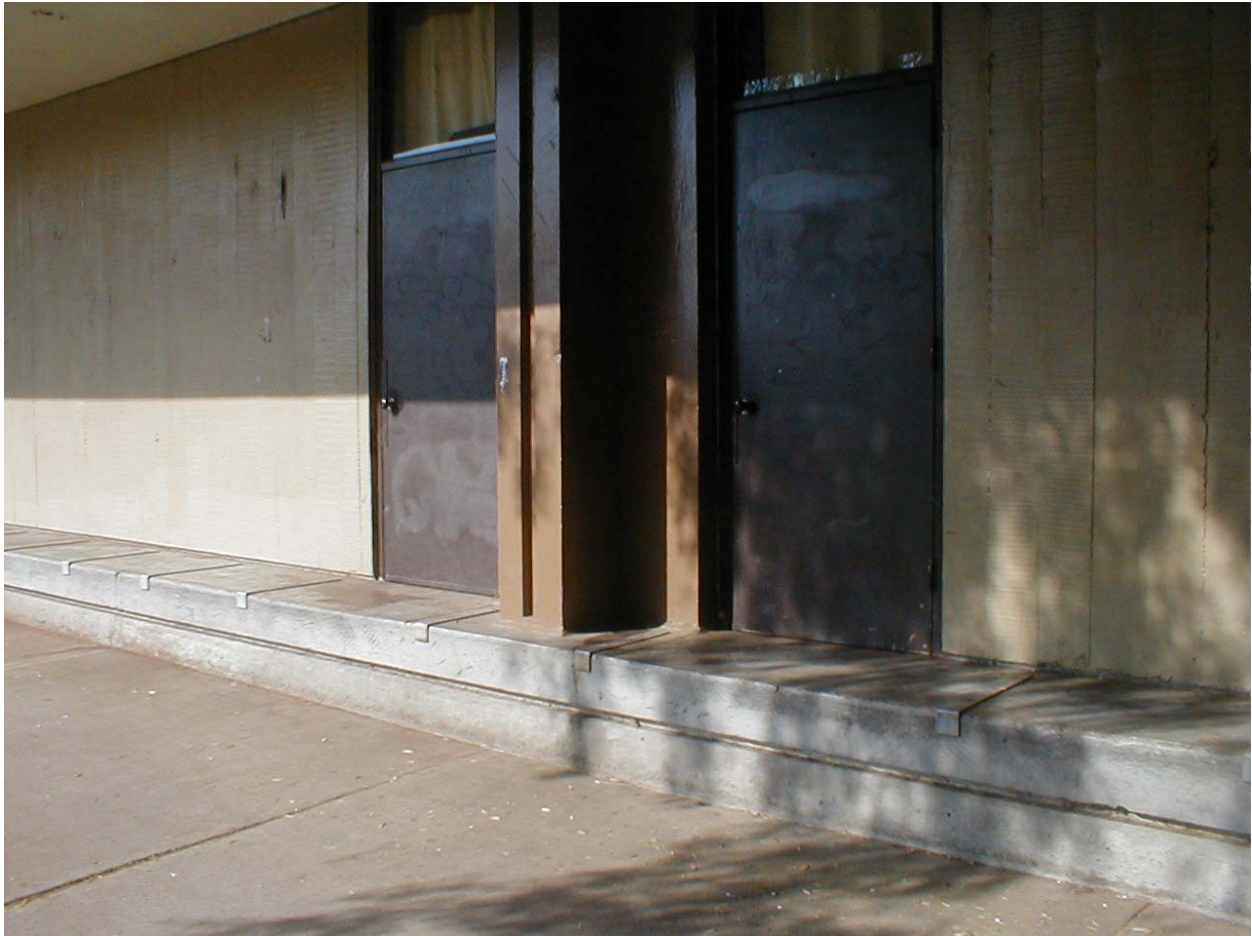
Nonconforming exit door at Mt. Pleasant High School.
