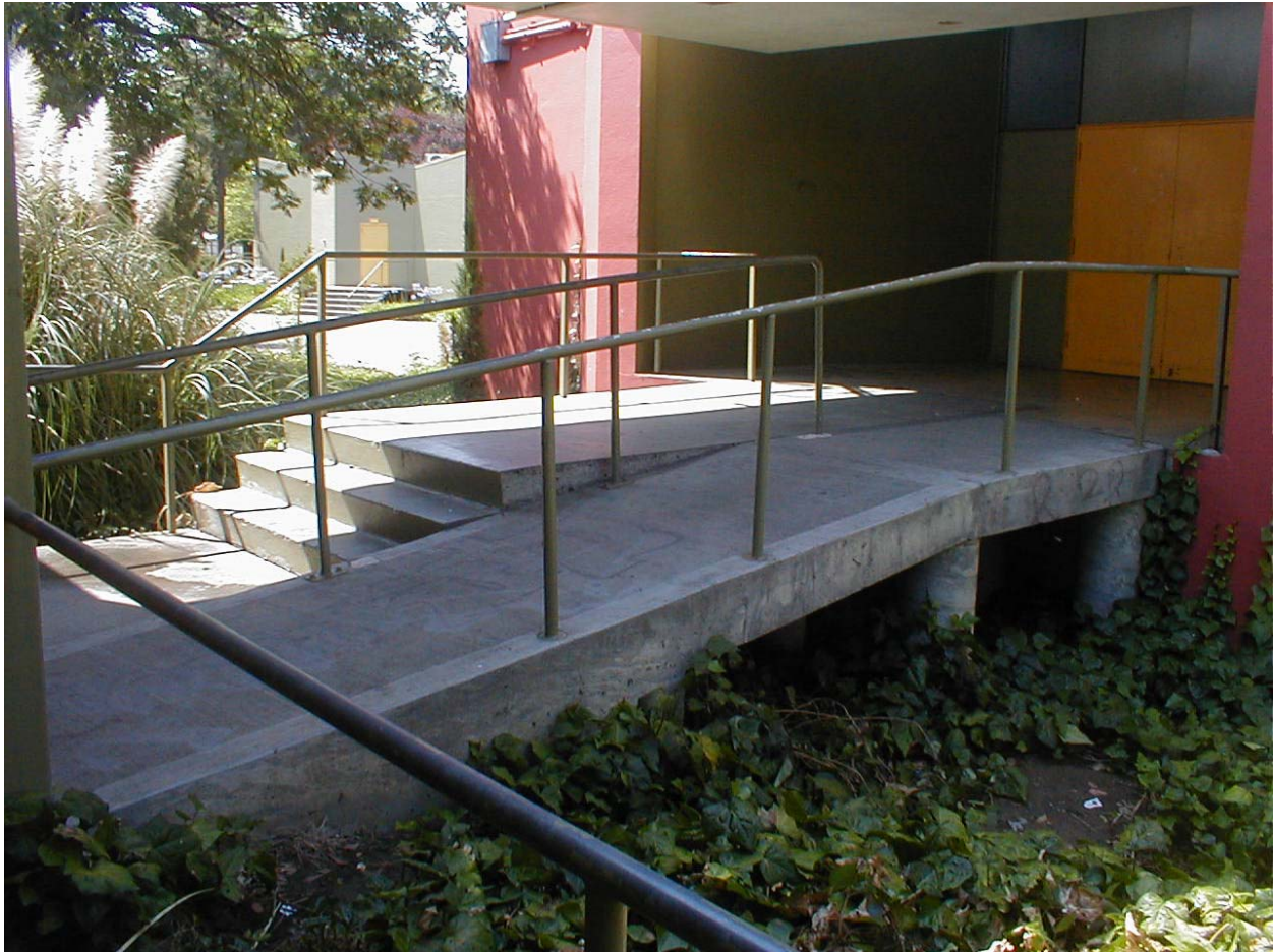
Nonconforming ramp at W.C. Overfelt High School.
