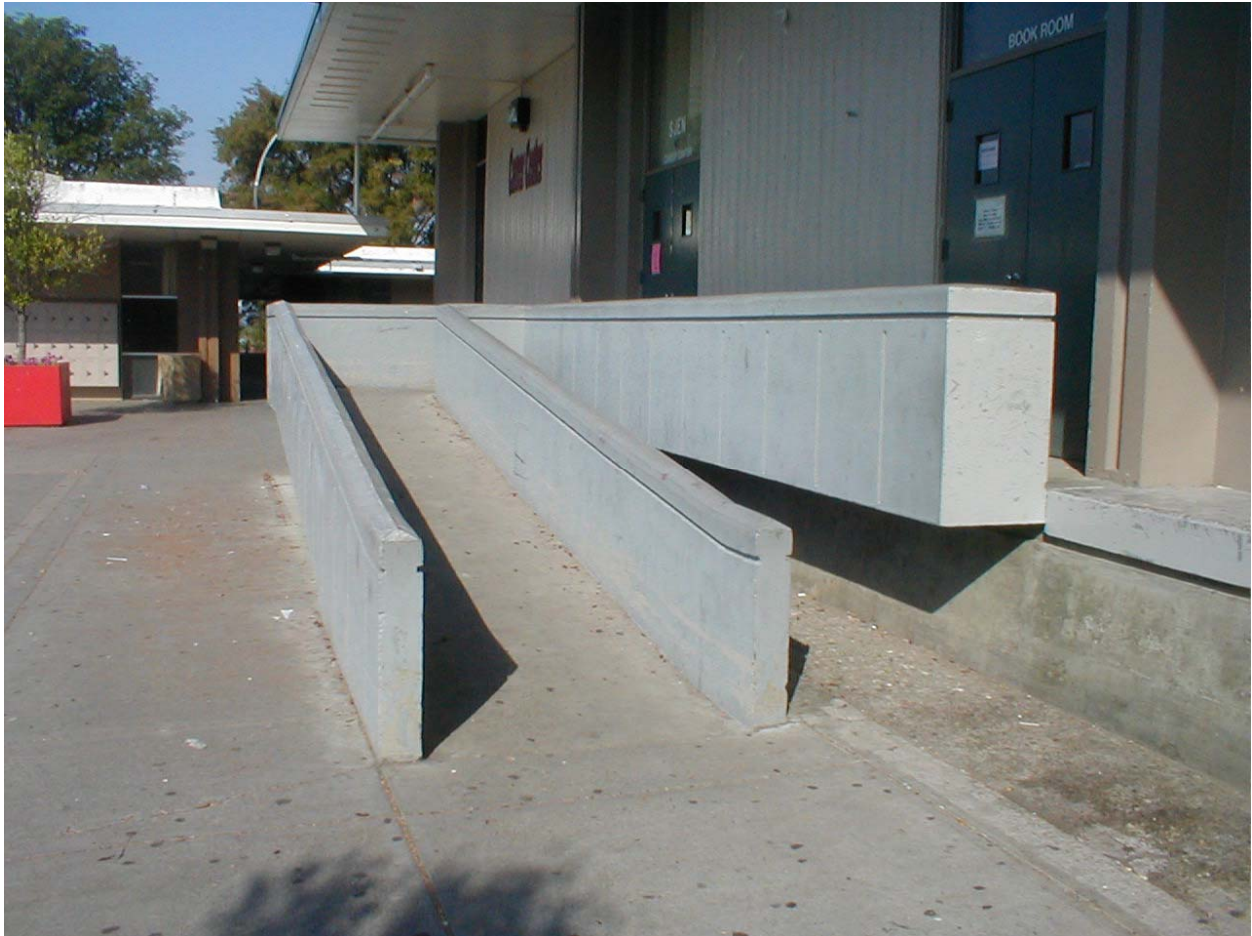
Nonconforming ramp at library of Mt. Pleasant High School.
